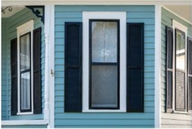
The black color of the storm windows makes them stand out against the white window frames and sash. The shutters are not operable and do not fit the window openings.
