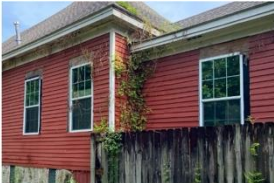
The vinyl replacement windows do not fit the existing window openings. Original window casing has also been removed.
