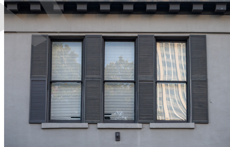
These shutters are inoperable and would not fully cover the windows if closed.
