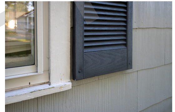
Do not install shutters flush with the siding material, as shown above.
