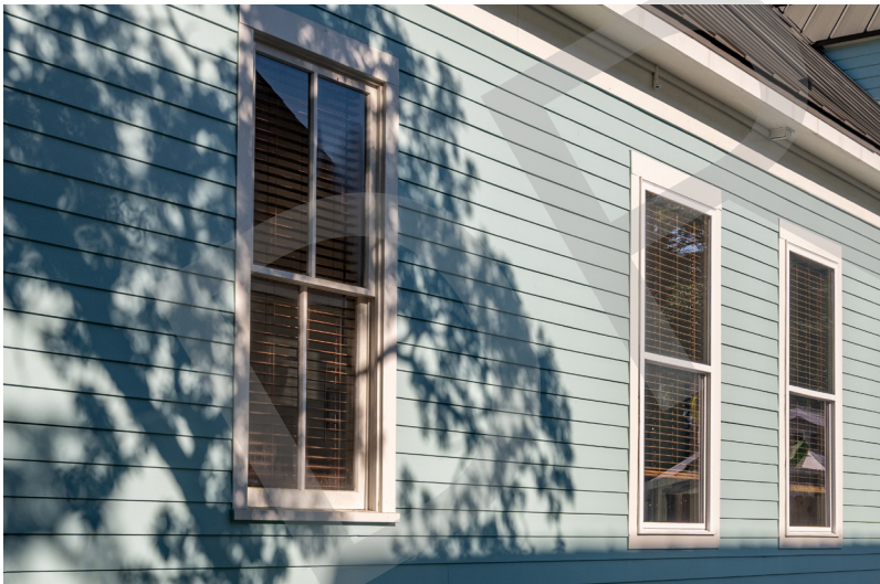
The two vinyl replacement windows (right) do not replicate the depth and dimensionality of the double-hung wood window (left).
