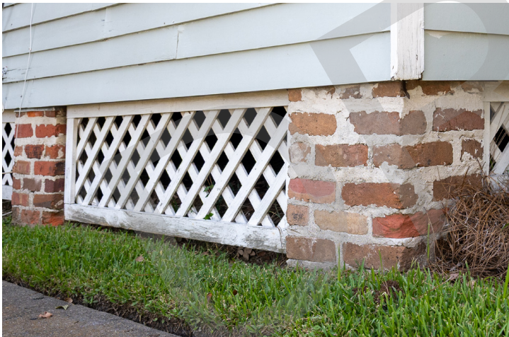
The lattice infill show above is properly framed and hung below the wood siding.
