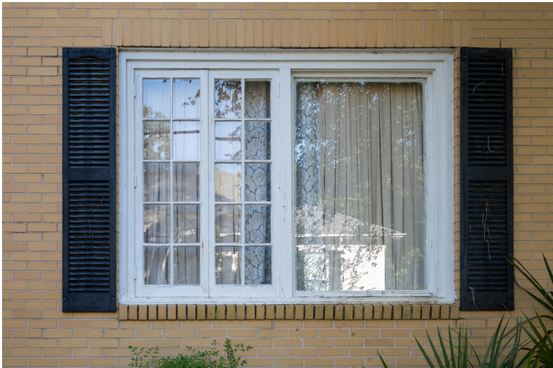
A fixed picture window (right) has replaced an original casement window that would have matched the remaining casement (left).
