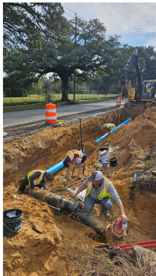
Construction is now underway on Martin Luther King Jr. Avenue from Broad Street to Butchers Lane.
